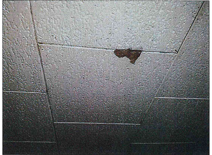
4/19/2016 SAMPLES S27 & S28 - 12X12 CEILING TILE FISSURE PATTERN NAIL ON Pic (56).jpg
