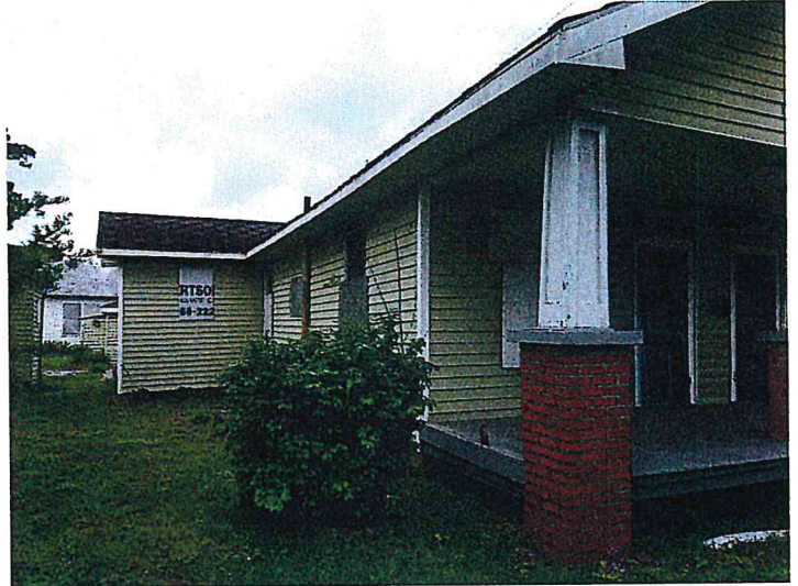
4/19/2016 EXTERIOR SIDE B - 521 A&B NE EVANGELINE THRUWAY Pic (40).jpg
